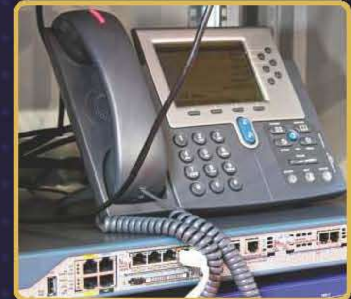
TELEPHONE EXCHANGE & BROADBAND
