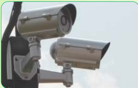
Security CCTV Access
